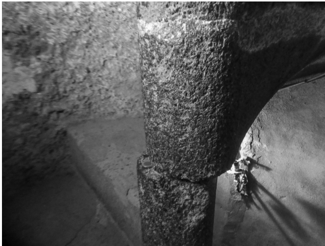
Figure 4. Displaced steps of the spiral staircase in Nagyvázsony donjon. A coin with a diameter of 24 mm for scale. #0376
