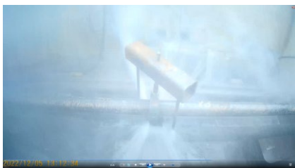
Y8 pipeline section
