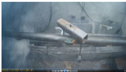
Y10 pipeline section
