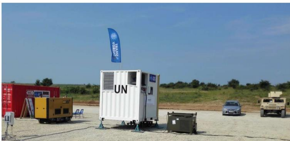
Figure 1. Prepared electrical network details on the CL15 international logistics exercise. 7
