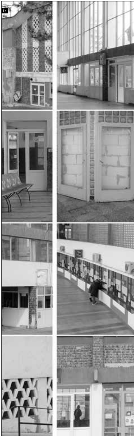
■ Photo 1.b. Photos of the main damages and alterations © Cristina PURCAR, Virgil POP
