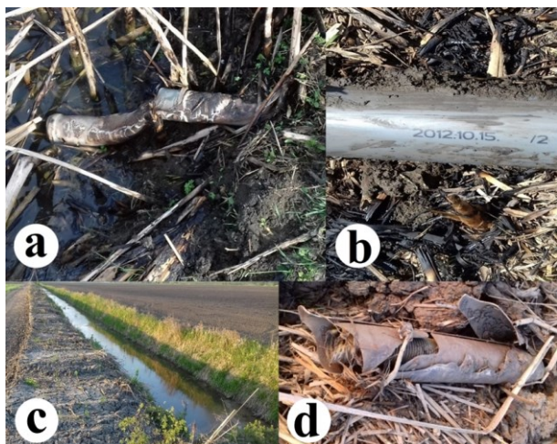
Fig. 7 Typical conditions of the drain pipes at the Mezőtúr study site: (a) melted PVC drain outlet in the channel side slope, (b) a few years old relocated drain pipe outlet, (c) open channel after sludge removal in Csanytelek, (d) ruptured drain pipe in spreaded sludge
