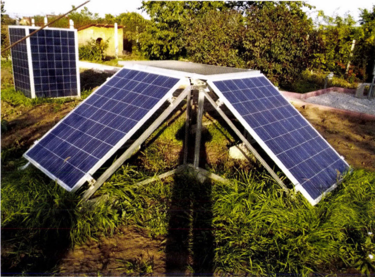
Fig. 2. The PV arrays at the station.
