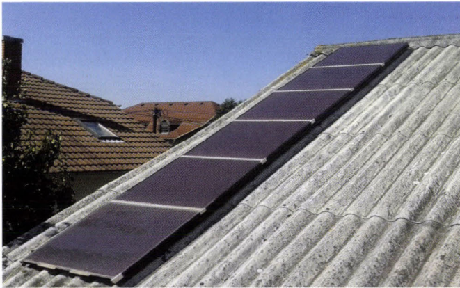
Fig. 6. Amorphous silicon solar panel on the roof.
