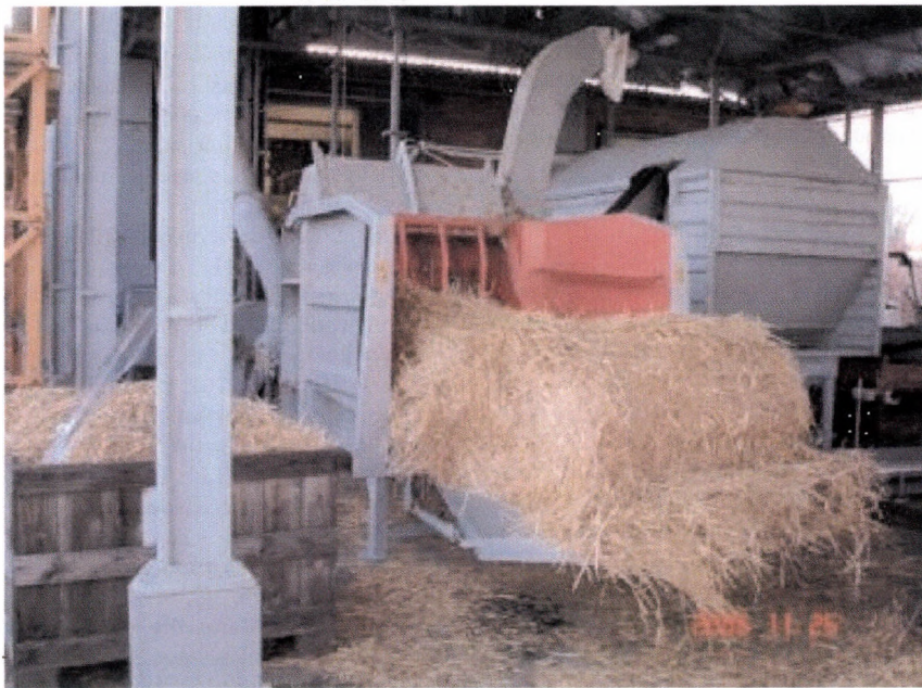
Figure 3. T&T Technik Ltd. agripellet plant, bale-opener, wheat straw before the grinding process
