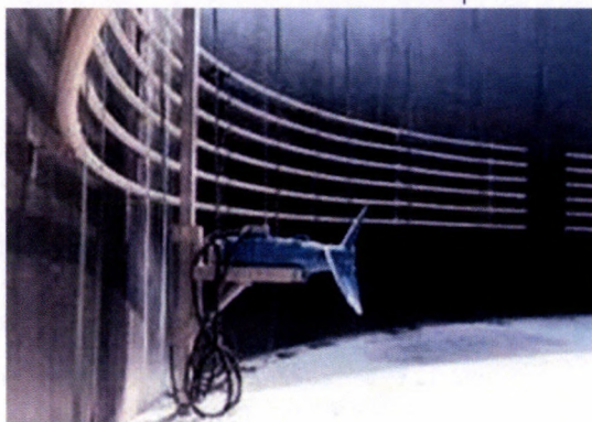
Figure 5. Small mixers (k 1 ) and installation scheme Vh – vertical setting, Hm – horizontal setting, Hs – heating tubes
