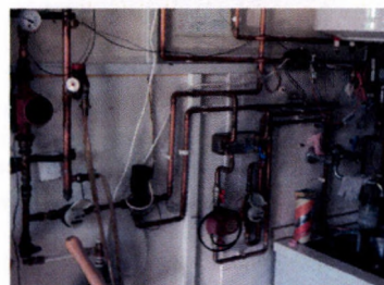
Figure 2. The tube and valve system inside the research laboratory
