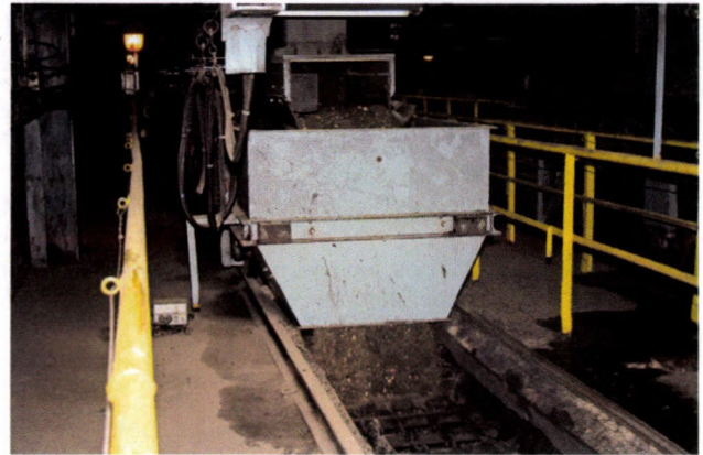
Figure 7. The system of boiler feeding with the coal and biomass mixture
