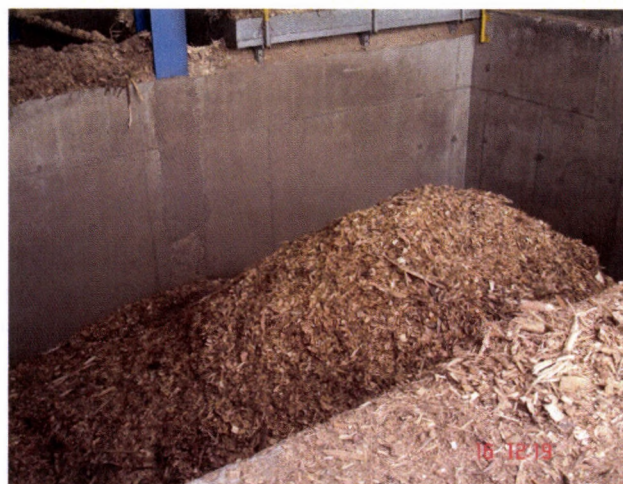
Figure 2. The hopper supplying the system of biomass feeding into the boiler
