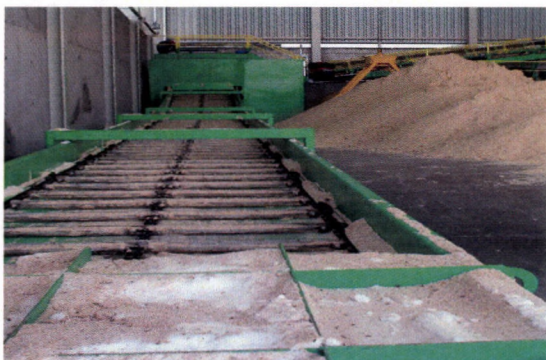
Figure 6. The biomass feeding system for the production of coal and biomass mixture for the cogeneration process.
