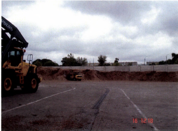
Figure 5. The storage yard for the biomass fed into the system supplying the power block.
