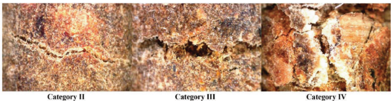
Figure 10. Photos of crack categories taken by digital microscope
