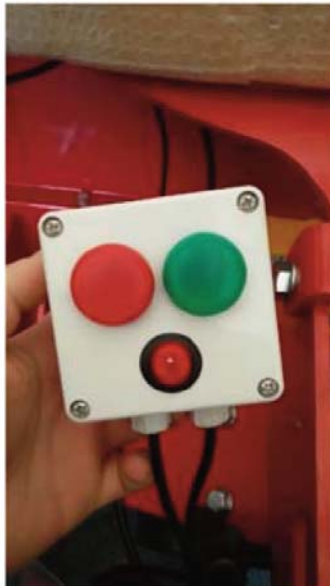
Figure 6. Control panel of INO Smart Hopper (Source: INO)
