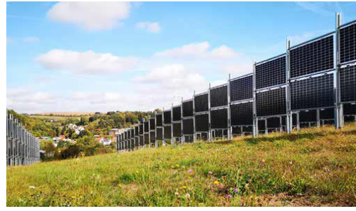
Figure 2. Bifacial modules installed vertically, Donaueschingen-Germany. @Next2Sun GmbH
