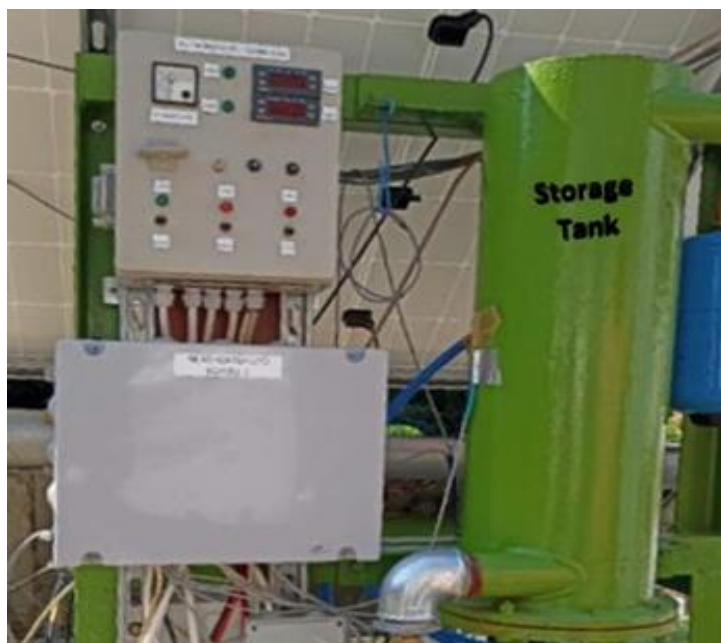
Figure 4. Arduino-based control unit and the storage tank
